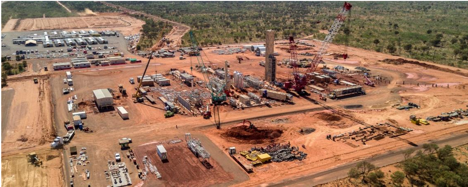
Above: Lifting is well underway at Jemena's Phillip Creek Compressor Station, near Tennant Creek. Image copyright Karl Heinz Herzog.
